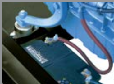
Rated battery capacity
